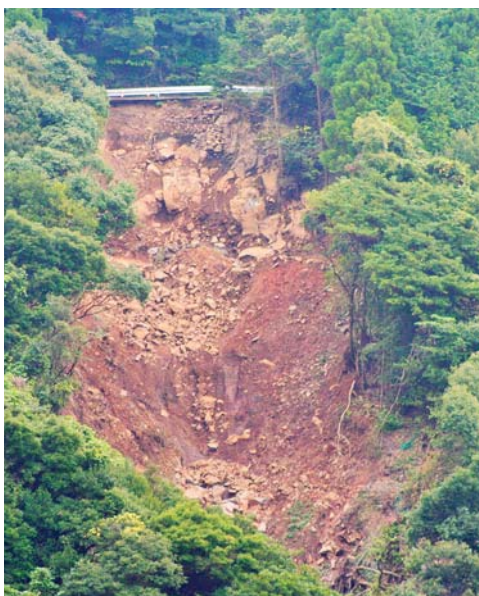
▲市道金松線路肩崩壊
